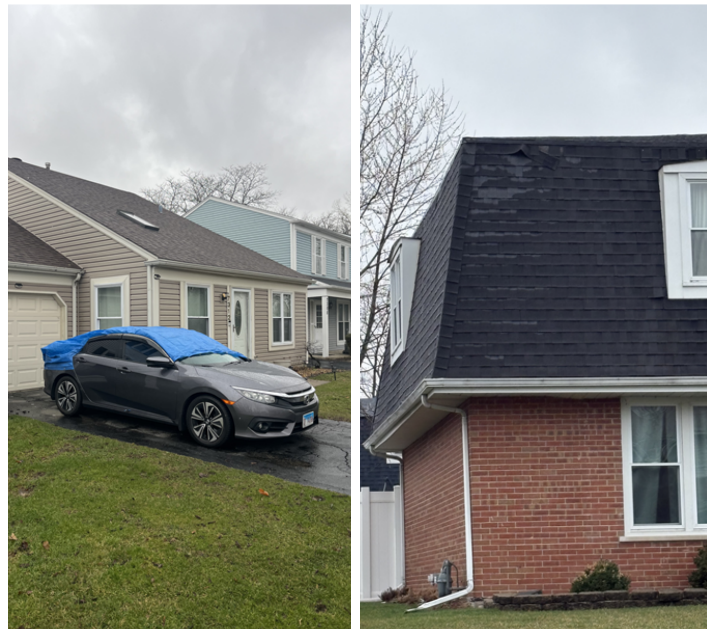
Damage Survey in the Chicago Area
